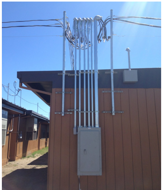
Power and utility connections for Interim Housing
